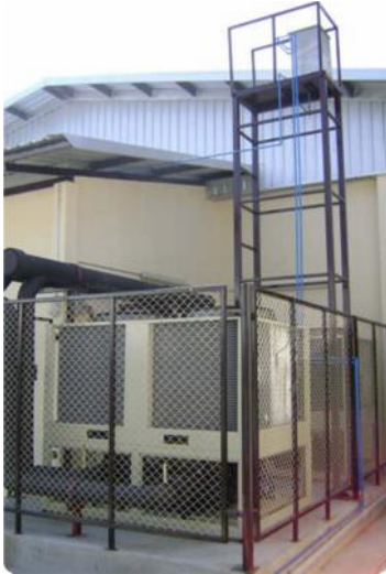
CHILLER AIR COOL
