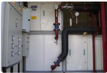
AIR HANDLING UNIT (AHU)
