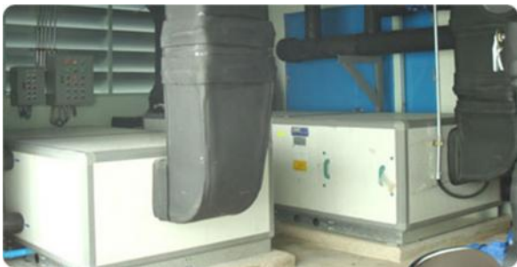
AIR HANDLING UNIT (AHU)
